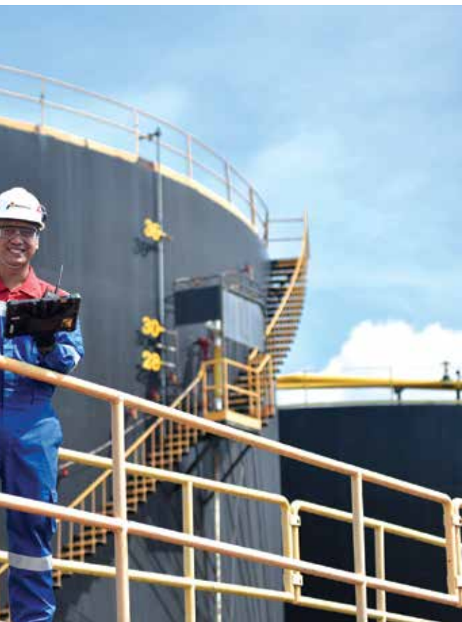
Pertamina Hulu Rokan workers walk around the Gathering Station #1 area while checking pipes in the Pertamina Hulu Rokan (PHR) area, Riau.
