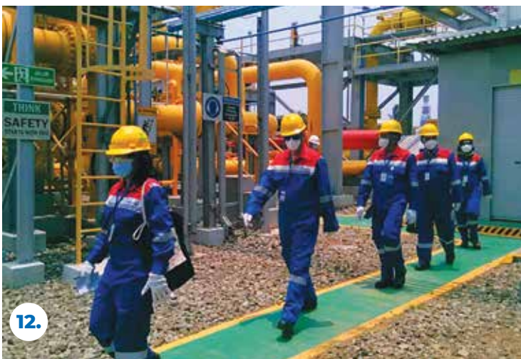
12. Kunjungan Komisaris Pertamina ke fasilitas penyaluran gas ORF Onshore Receiving Facility) Nusantara Regas di Muara Karang, Jakarta pada Selasa (12/10/2021). The visit of the Pertamina Commissioner to the Nusantara Regas ORF gas distribution facility in Muara Karang, Jakarta, Tuesday (12/10/2021).
