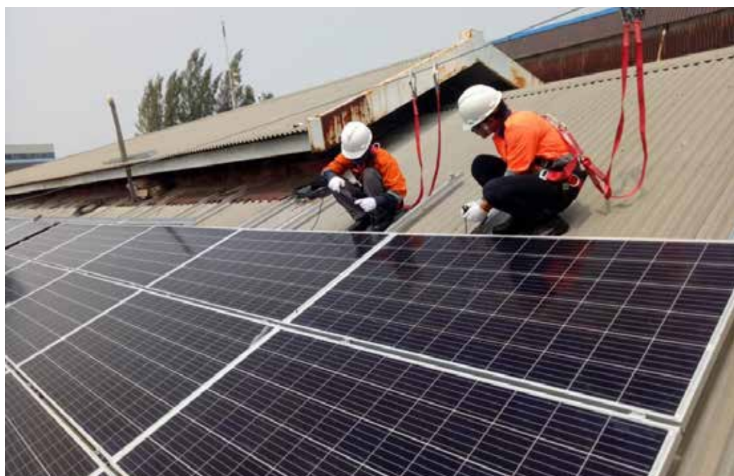
PLTS Logistics Building Pertamina International Shipping.
